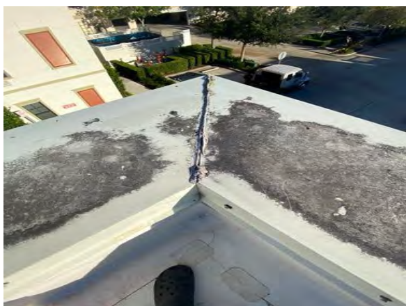
Some of the coping metal have openings where they connect.
