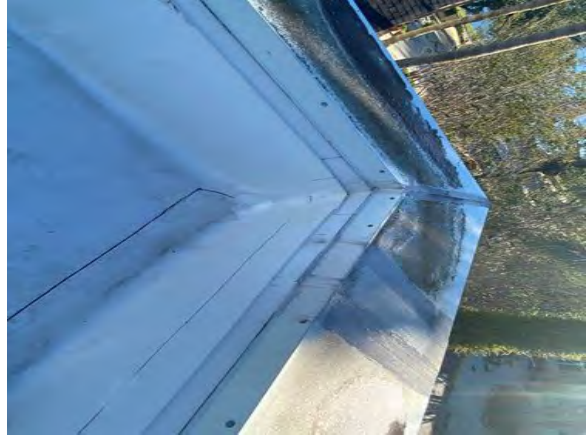
Angle change for the coping metal seems watertight as well as the walls
