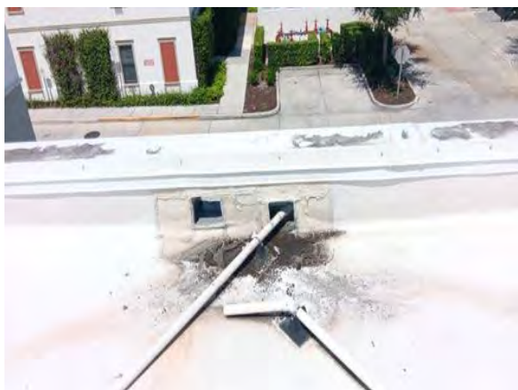
Condensate lines discharging water on roof.
