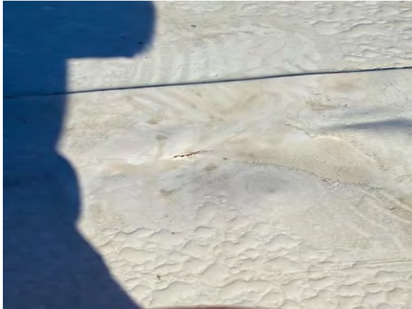
Hole to be repaired.
