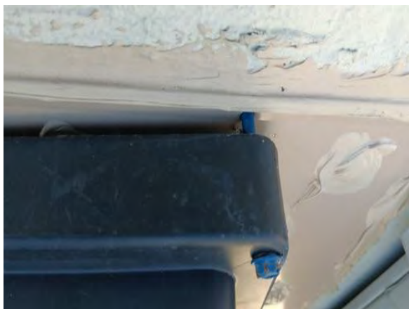
Scupper overflow fastener not sealed
