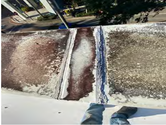
Opening on the coping metal where they meet. Could cause possible leaks in future.
