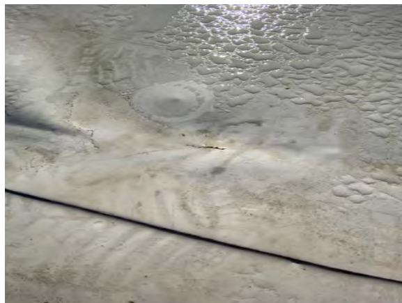
Possible opening that could cause leaks in the near future.
