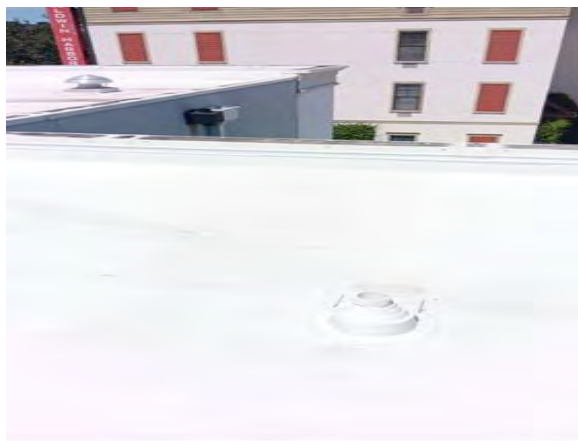
Angle change securement and pipe penetration.
